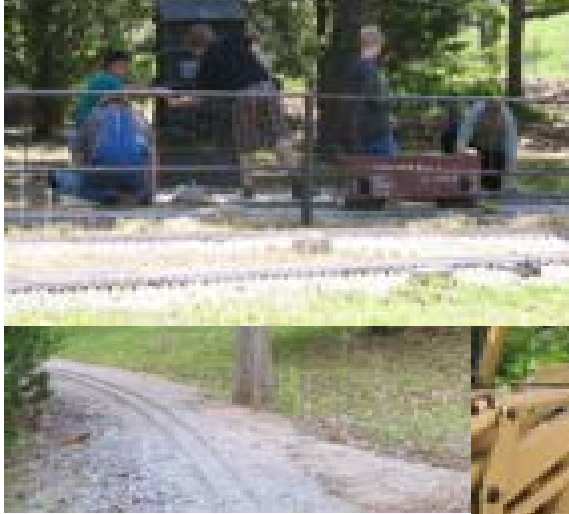
A track gang led by Christopher Lacock putting the final ballast touches to the No. 2 main through the passenger loading area.
